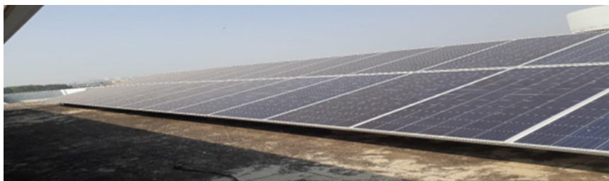
Fig. 1: Commercial sized solar arrays installed.
