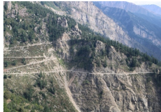
Plate 2: Landslide occurrence due to road construction resulted in fragmented pastureland nearby Thamoh village
